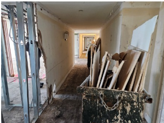
Photo of demolition inside the former JFK Hilton, which is being converted into a 318-unit housing complex for formerly homeless people and low-income New Yorkers. Photo courtesy of Aufgang
