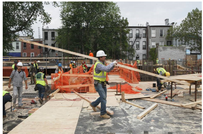
Workers at 470 Fourth Ave. in Brooklyn, one of eight projects by Aufgang Architects to receive building permits before Monday night's scheduled expiration of the 421-a tax break. PHOTO: ANDREW HINDERAKER FOR THE WALL STREET JOURNAL
